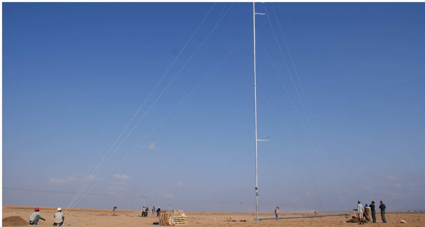
Ethiopia's first 40 metre wind measuring mast being erected in Aysha in January 2010. The certified mast was made possible through funds and technical know-how transfer from the PPP
